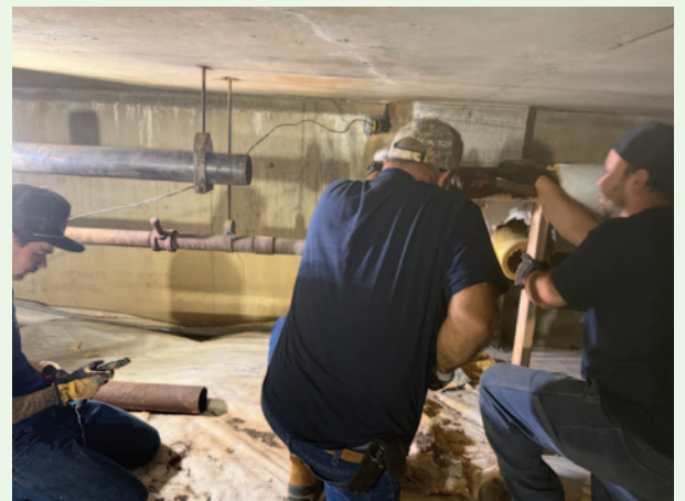
West Islip School District Maintenance members saving the district money, in lieu of using private contractors to repair the leaking steam pipes in Paul J. Bellew Elementary School. Local 237 members Troy, Tom, Matt and John took care of it all.
